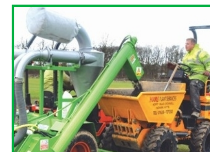
Discharges directly into dumper truck
